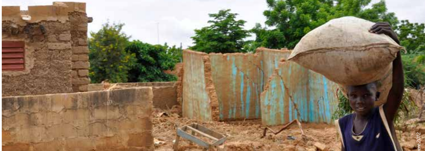
Floods resulting from climate change destroy infrastructures in Niamey, Niger.
